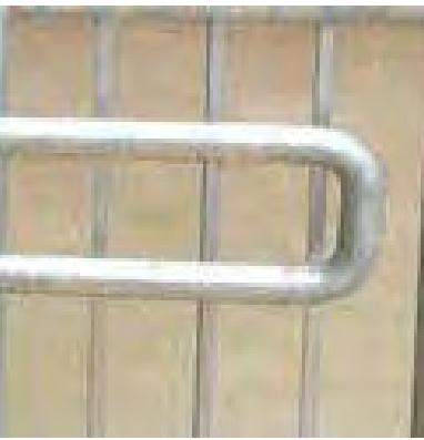
HR01 STAINLESS STEEL HANDRAIL
